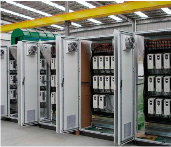
A total of 188 ABB standard drives are mounted side by side to save space.
