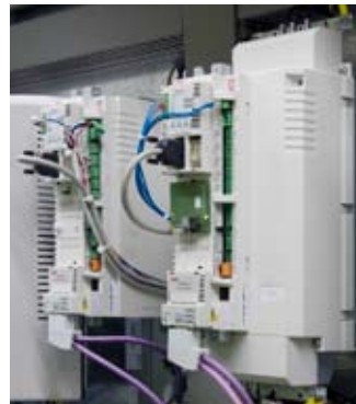
Three ABB high performance machinery drives of ACSM1 series were installed to the sheet cutter machine.
