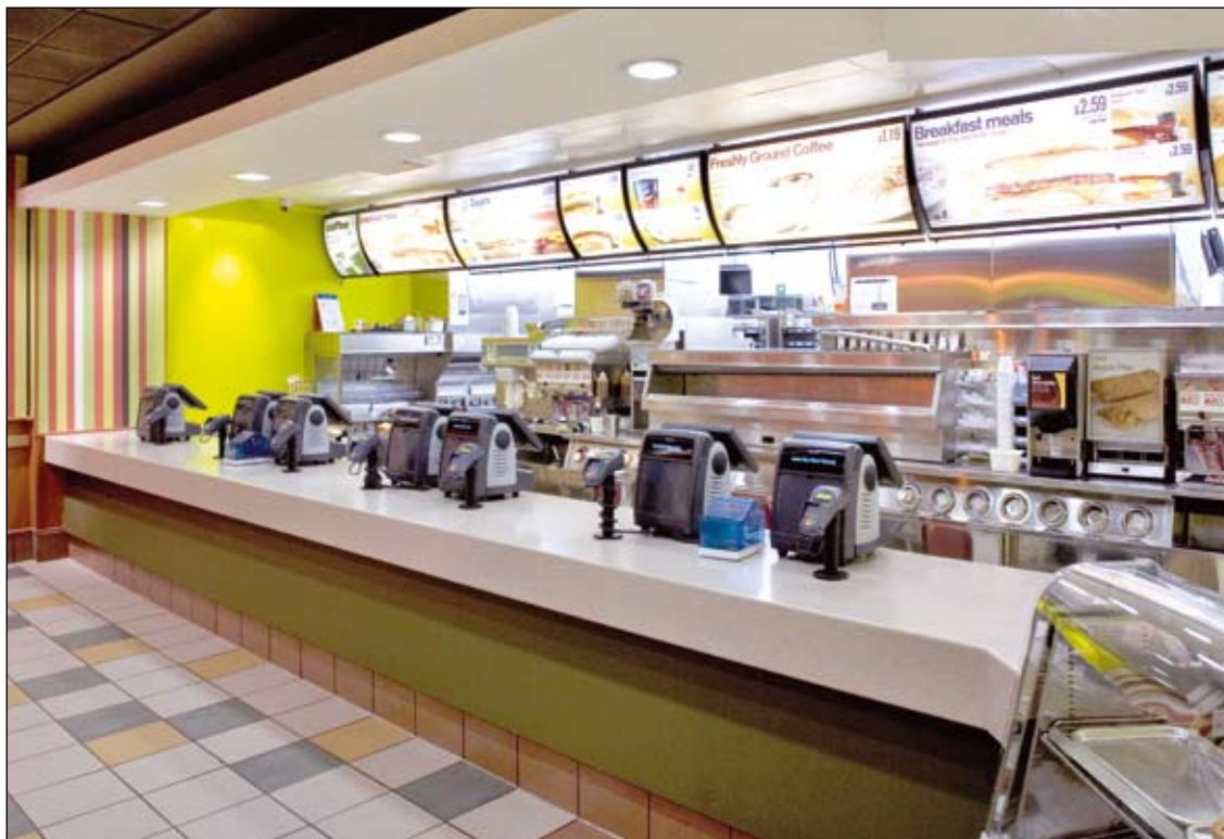
McDonald's restaurants throughout the UK are using ABB standard drives for HVAC to save energy and control cooking odors.
