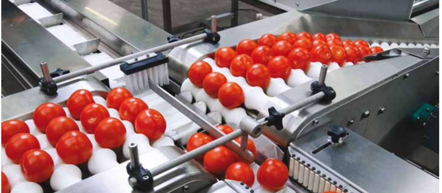
ABB high performance machinery drives control the speed of the tomato handling conveyors.
