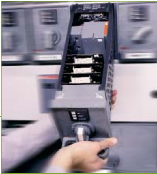
MCU mounted in withdrawable MNS drawer 8E/4. MCU executes control commands from and reports status to remote control systems.
