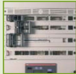
Integrated Tier Switch (ITS) SlimLine fitted in MNS LV switchgear
