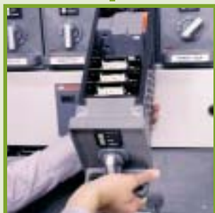
Motor Control Unit (MCU) in Motor Starter
