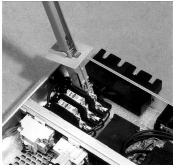
Replacing of fuses in 2M units takes place with the unit removed from the cubicle.
