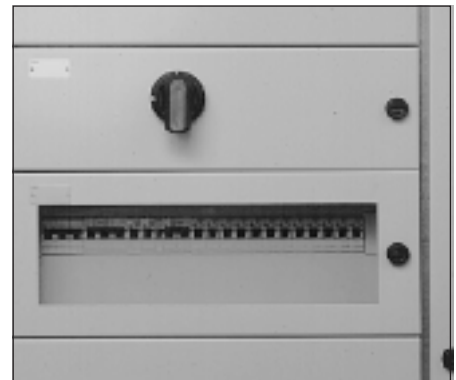
MCB-unit with back-up MCCB.
