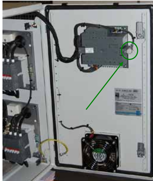
Figure 10: Location of thermal cutoff switch in APC03
