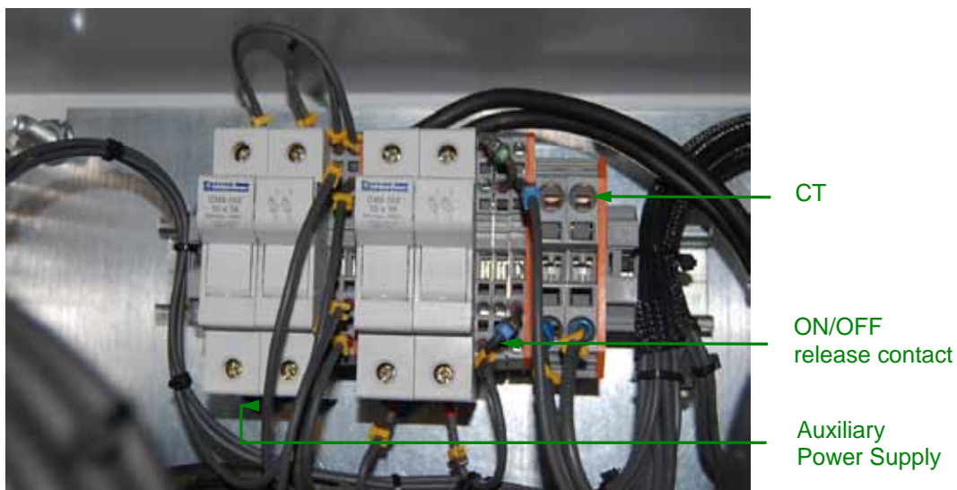
Figure 19: APCL03 cables connection
