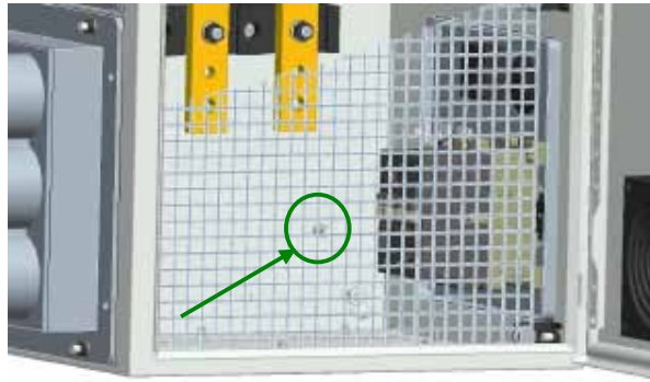
Figure 14: Earth connection in APCL03
