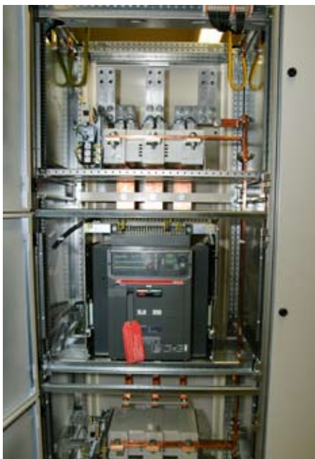
Incomer 3200A with air Emax circuit breaker and two earthing switches
