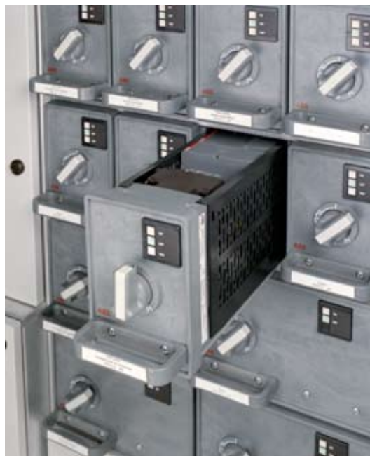
Switchboard example with withdrawable modules. One partly withdrawn, others in TEST position
