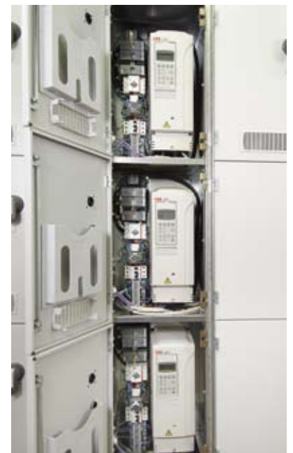
Frequency converters integrated into the MNS system
