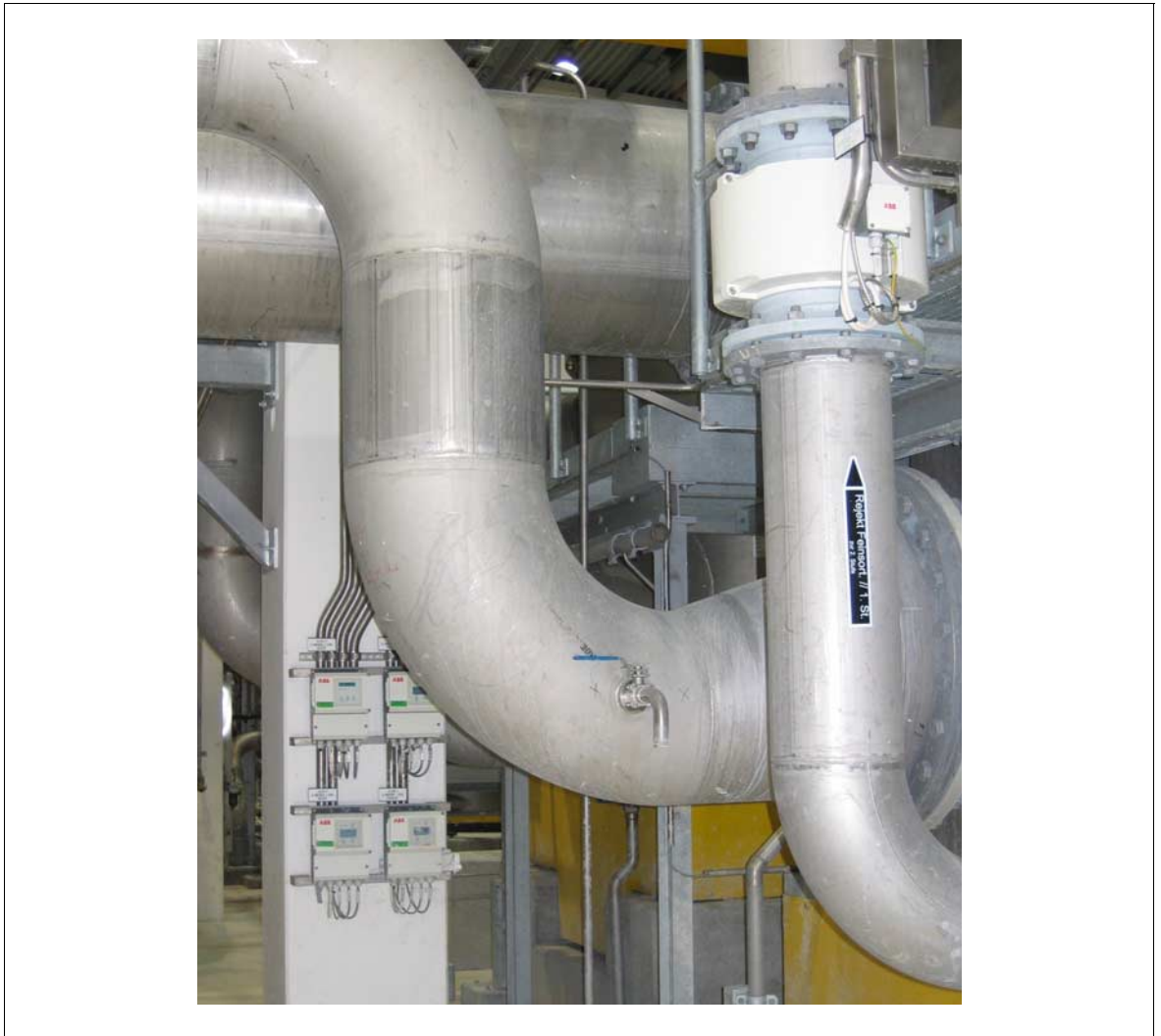
Fig. 1-1: Electromagnetic flowmeter in stock preparation
