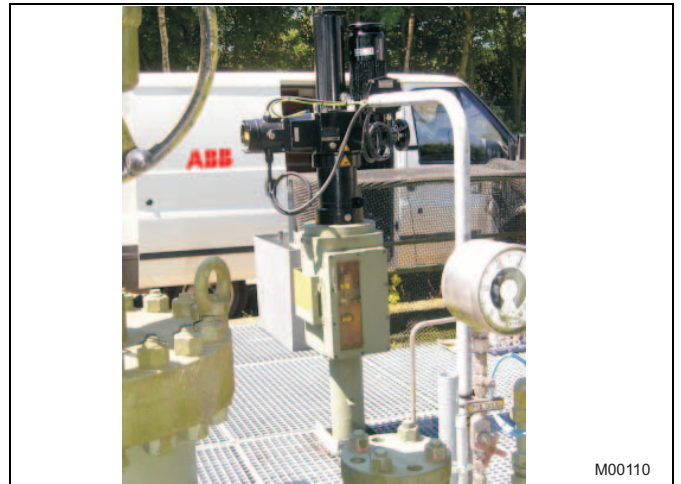
Fig. 39: Commissioning support from specialist ABB personnel during installation of an explosion-proof linear actuator RSDE10
