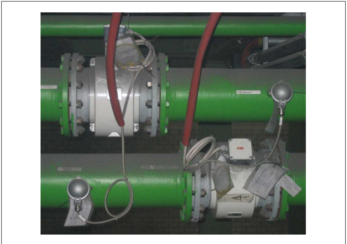
Fig. 2-1: E. g.: Electromagnetic Flowmeter in the cooling water supply and return lines including temperature measurements
