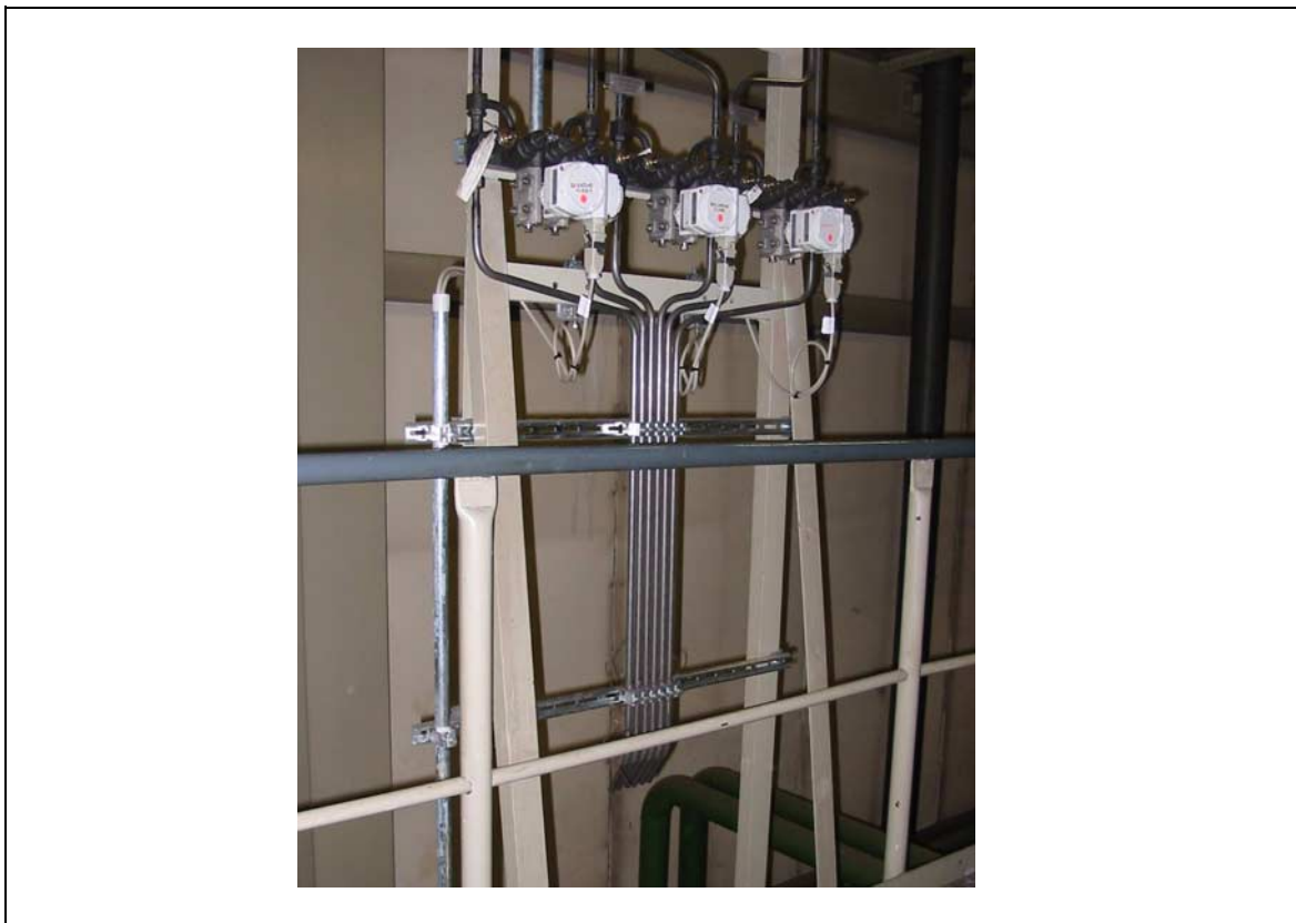
Fig. 4-1: Transmitter instrumentation with 5-fold valve combination and blowout pipes for steam measurement
