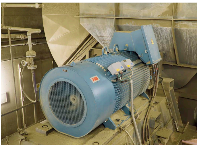
The clinker cooler exhaust fan motor controlled by ABB's ACS 2000 variable speed drive.
