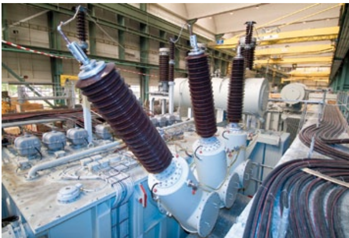
View of a converter transformer
