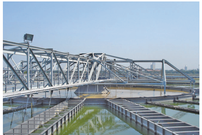
Clarifier at MWA’s Bangkhen water treatment plant
