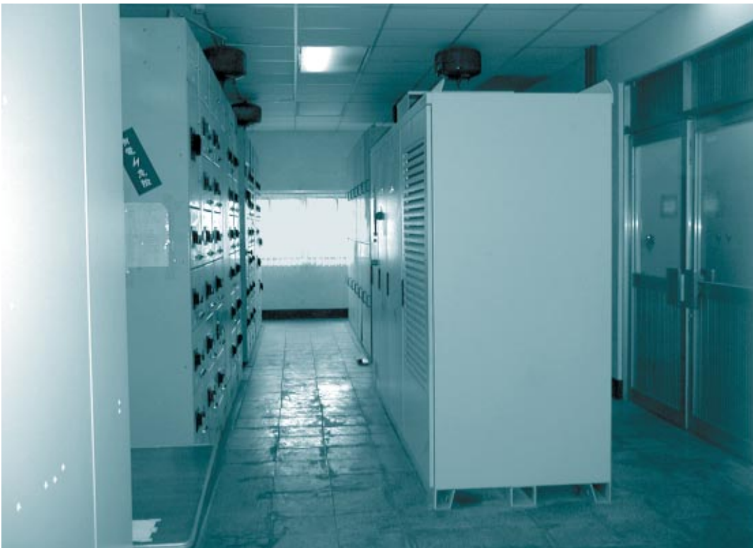
View of one ACS 1000 drive (on the right) installed at CSC.
