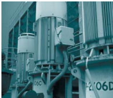
View of booster pumps.
