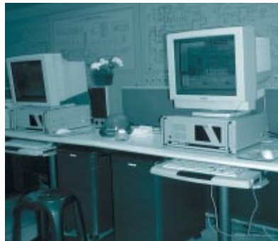
View into the control room.
