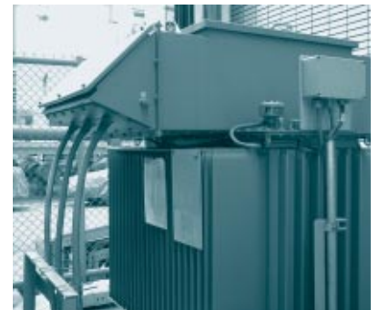
View of one isolation transformer.
