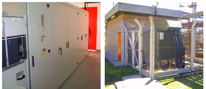
View of motor driven by ACS 1000; ACS 1000 in converter building; Converter building and three-winding input isolation transformer.
