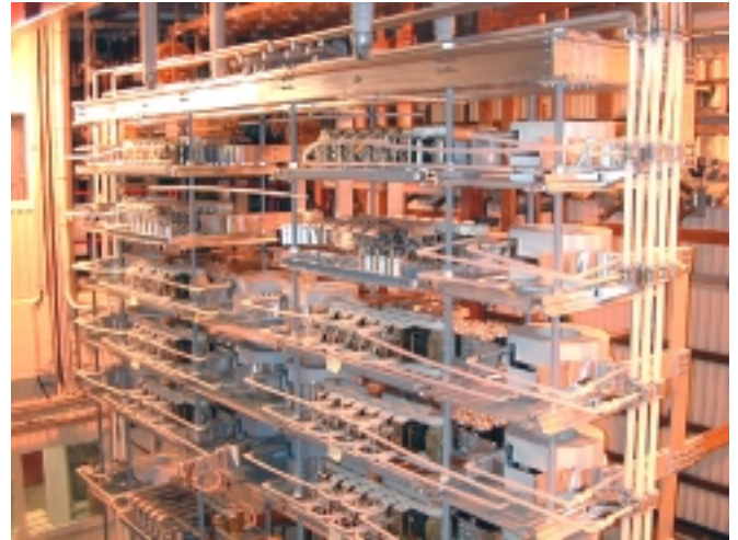
Fig. 2. View of six-pulse back-to-back bridges and test object
