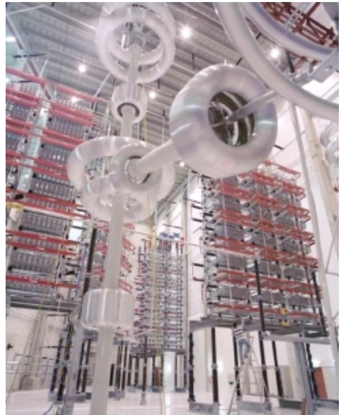
Fig. 3. Capacitor banks of the voltage section
