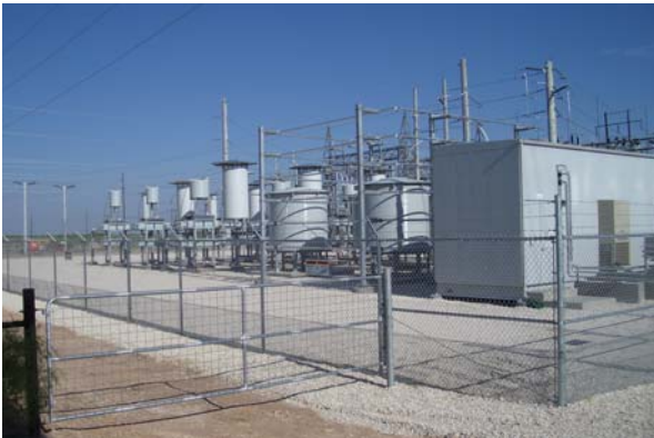
Fig. 9. Crane 69 kV, -40/+50 Mvar SVC.
