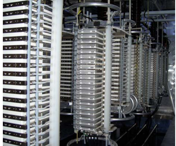
Fig. 16. SVC Light valve assembly.
