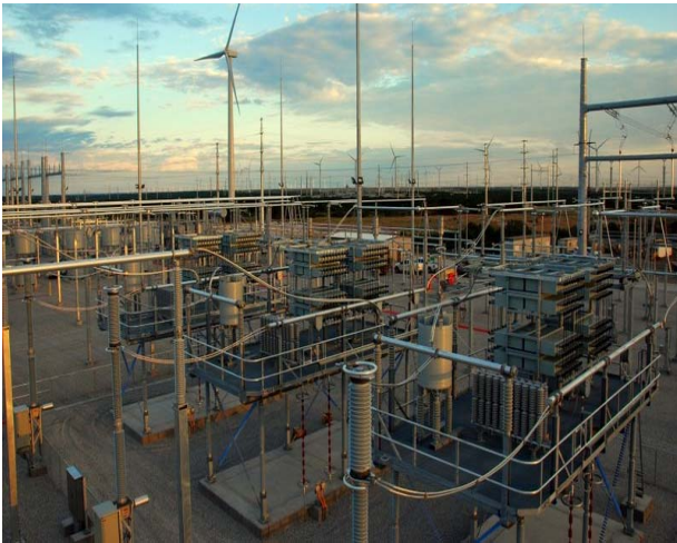
Fig. 12. Wind farm and 345 kV Series Capacitor, Texas.
