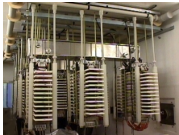
Figure 5: Photograph of SVC Light valve.
