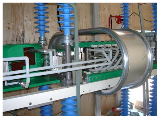
Fig. 3 Saturable reactor and thyristor module assembled in an enclosure installation
