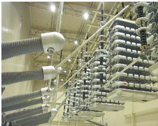
Fig. 5 Suspended valve installation at LongQuan converter station of Three-Gorges — ChangZhou HVDC transmission project
