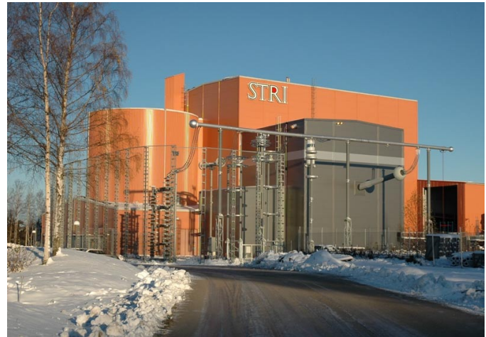
Fig. 1. 800 kV HVDC long term test circuit installation at STRI, Sweden.
