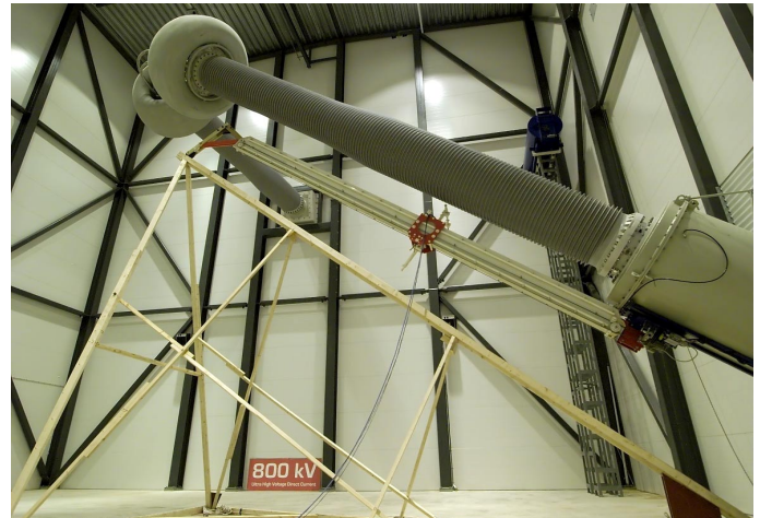
Fig. 9. Measurement of 2-dimensional DC electric field along transformer the bushing, during the long duration test. The wooden structure is used to put the robot in parallel with the bushing. The position of the probe is indicated by the red circle and it is remotely moved along the bushing.
