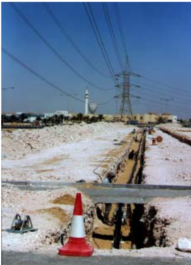
Figure 7: Example of cable laying in a corridor already used by OH-lines. AC PEX-cable in Qatar.
