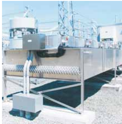
Dry air blast cooler
