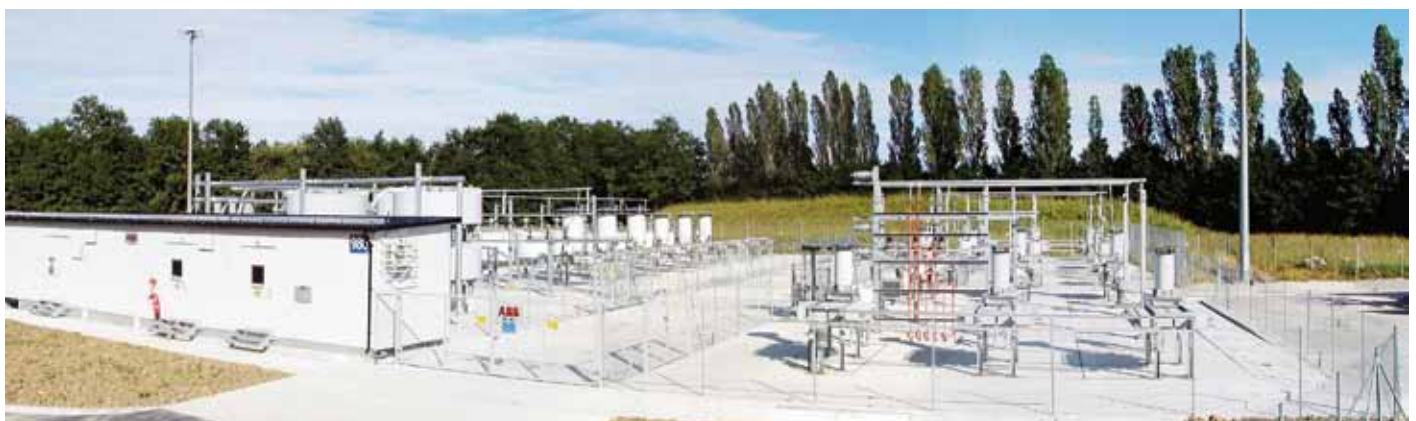
SVC for voltage stabilisation of a large pulsating load.
