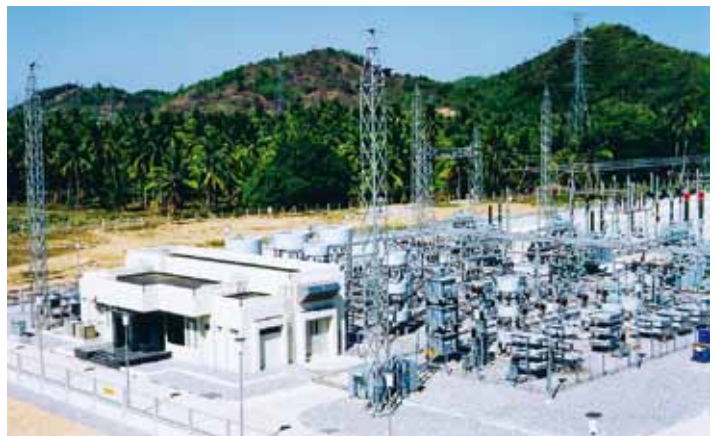
This SVC has boosted power transmission capacity by over 50 percent in a 230 kV system.
