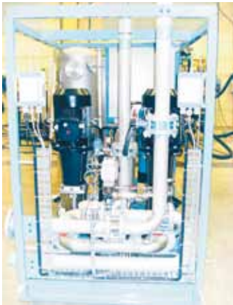
Cooling water pump unit
