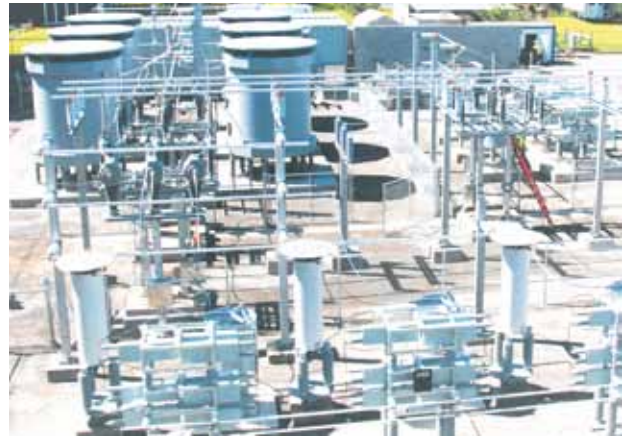
Directly connected SVC
