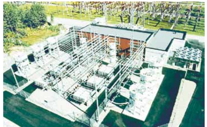
The SVC is an excellent tool for achieving dynamic voltage control of power systems.
