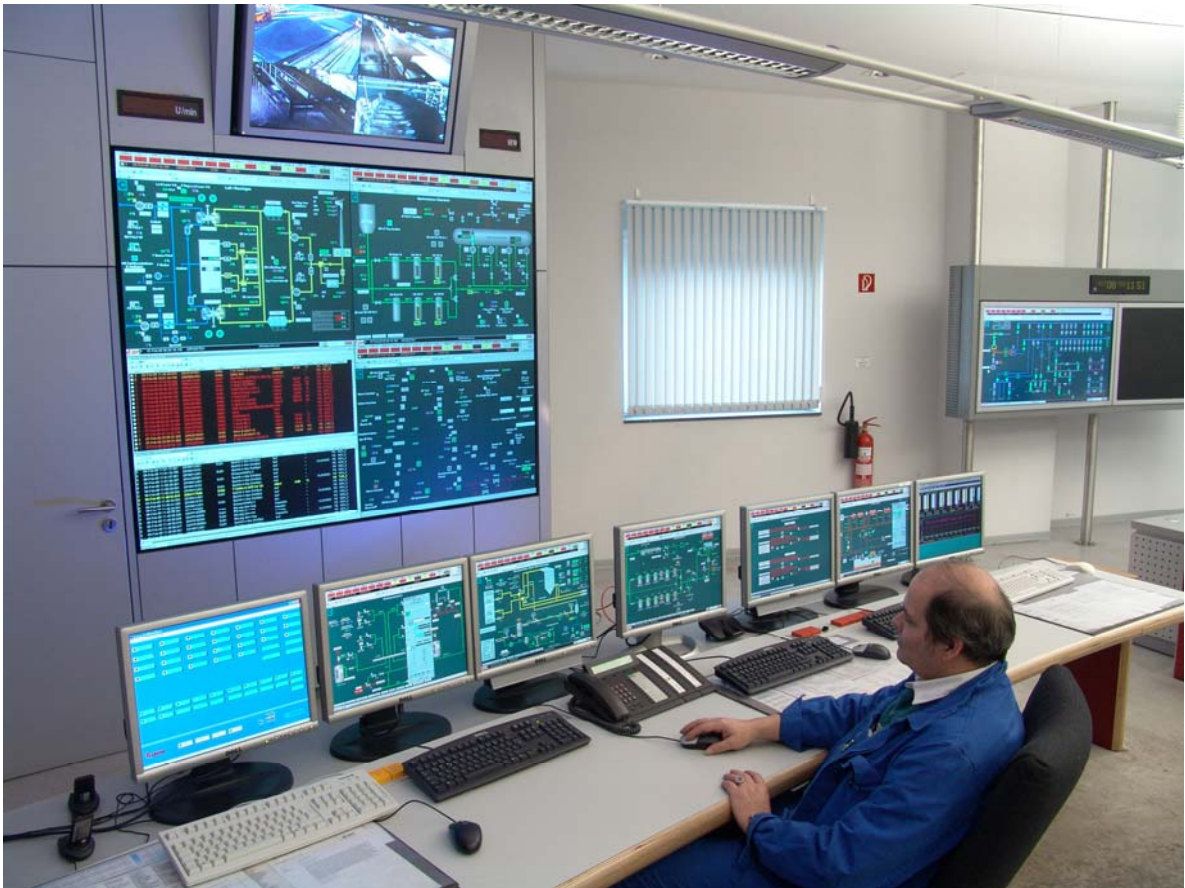
Control room of Unit C
