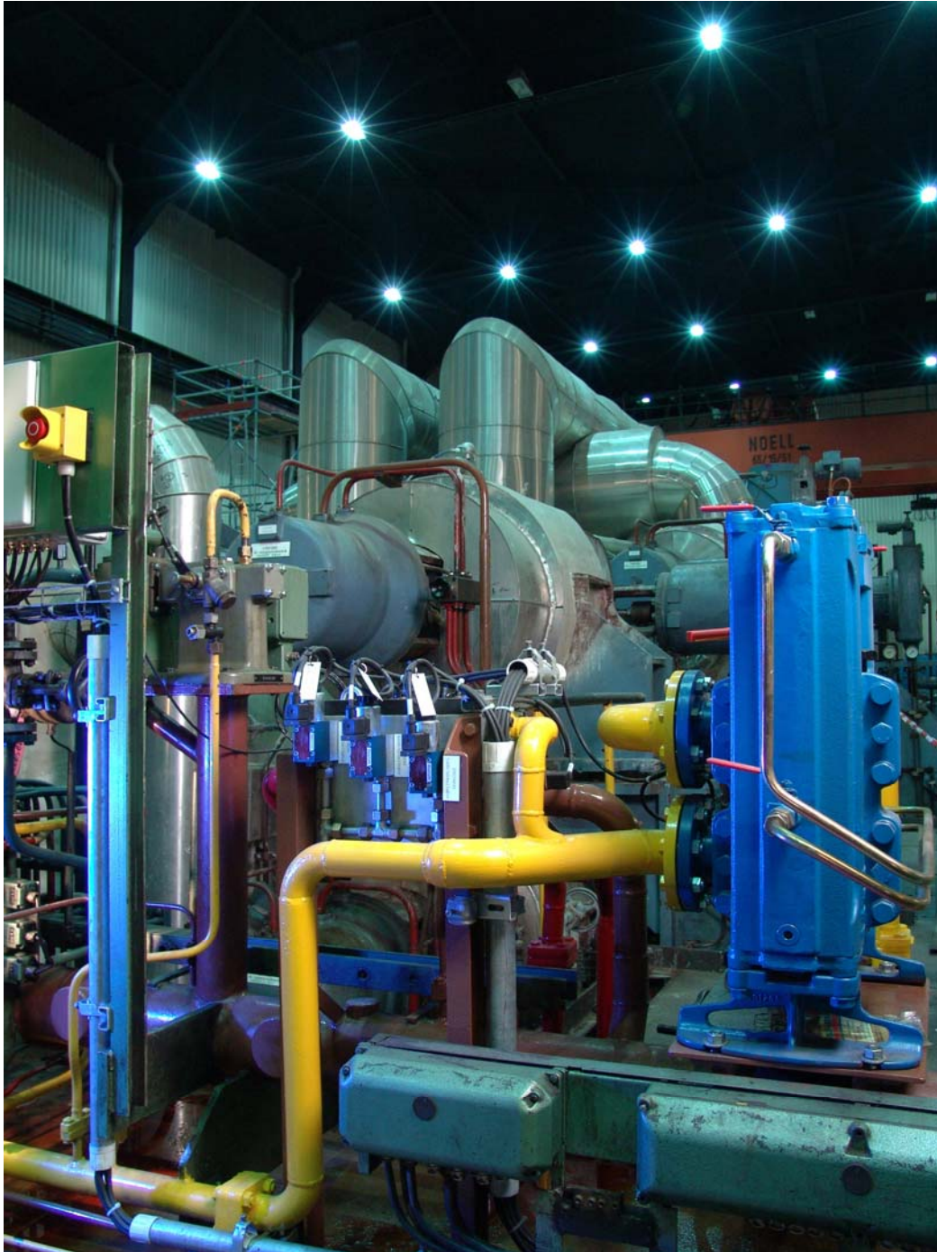
Turbine hall of Unit C – parts of the hydraulic system modified by ABB in the front
