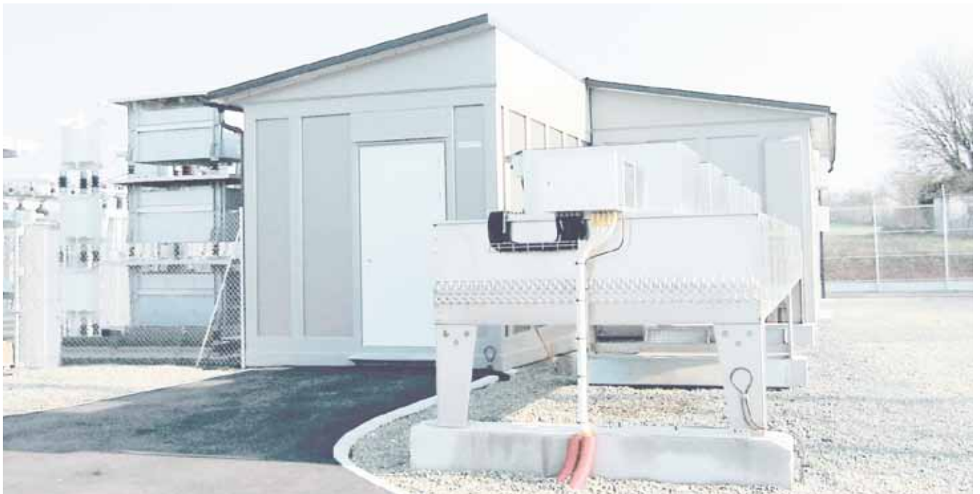
Fig. 1: SVC Light for railway load balancing
