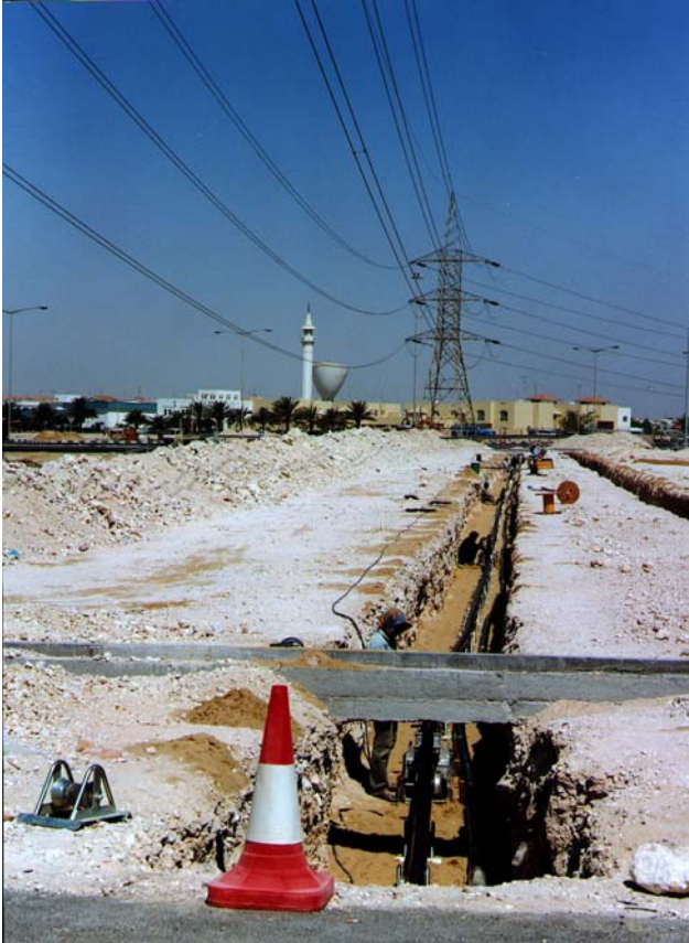
Figure 5: Example of cable laying in a corridor already used by OH-lines. AC PEX-cable in Qatar.
