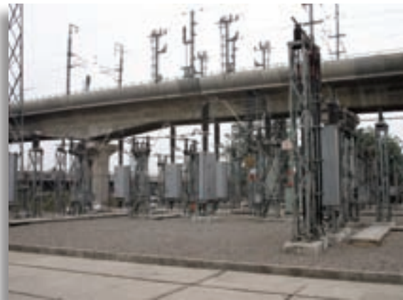
25kV Traction substation, Feeding post and Pole mounted Interrupters
