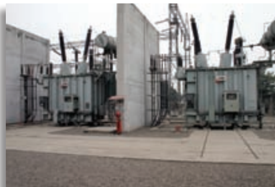
220/27.5kV Traction Transformers
