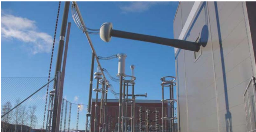
Fig. 1. 800 kV UHVDC outdoor equipments in long term test circuit installation at STRI, Sweden.
