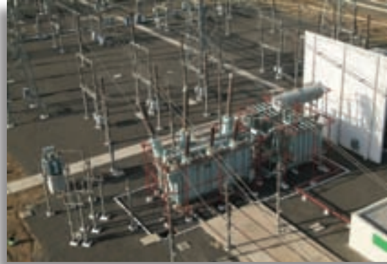
400/220 kV three phase 315 MVA Auto Transformers
