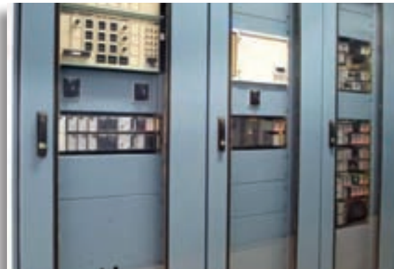
Control and Relay Panels
