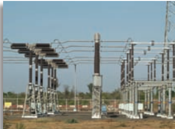
400 kV Circuit Breakers, Current Transformers and Disconnectors
