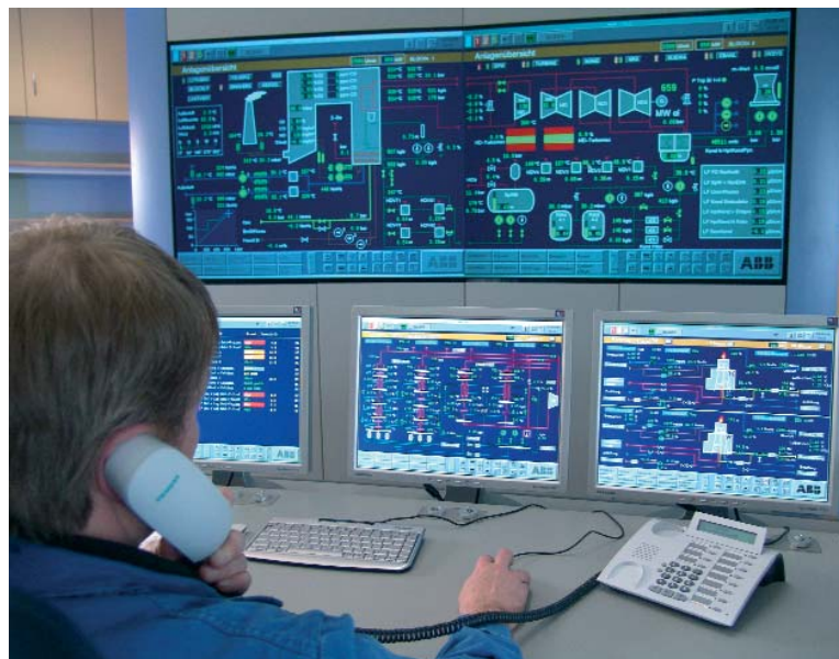
Staudinger power plant unit 4, Germany
