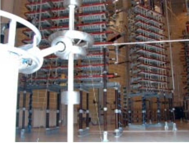
Fig. 6 Capacitor banks in the voltage circuit
