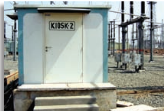
Outdoor AC Kiosk for Substation Automation panels
