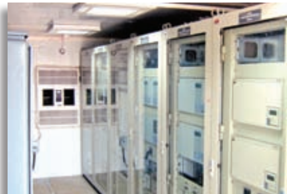
Substation Automation panels inside the AC Kiosk
