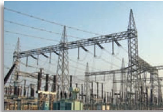
400kV Switchyard with 800kV Tertiary Transformer
