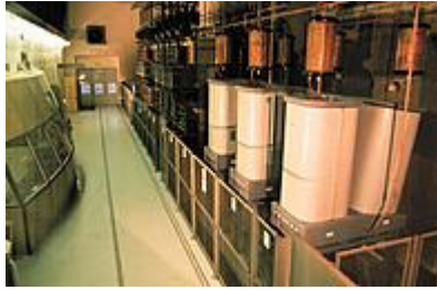
The first HVDC thyristor valve group in the Gotland link
