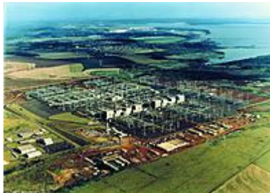
Foz do Iguaçu converter station in the Itaipu 6,300 MW transmission.
