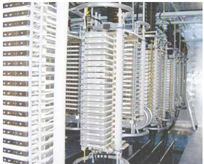
Converter valve assembly.
