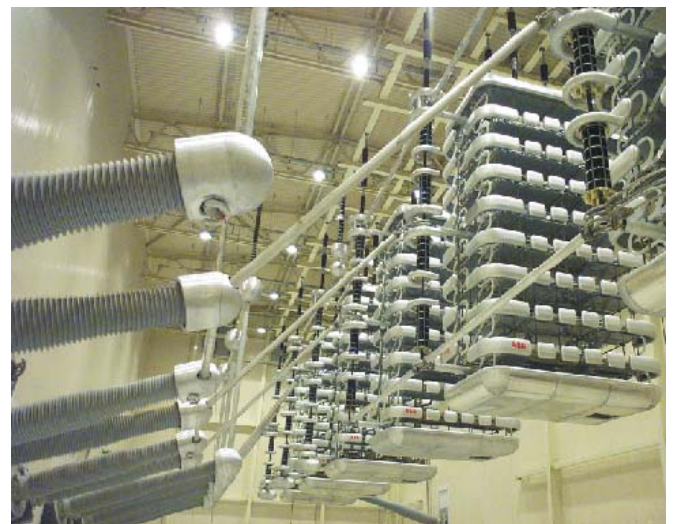
Fig. 1 Valve structure and installation at Longquan station (Three-Gorges – Changzhou HVDC transmission)
