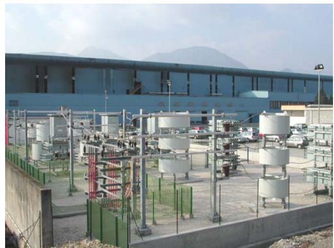
Fig. 5: Site view of the SVC at Ferriere Nord, Osoppo.
