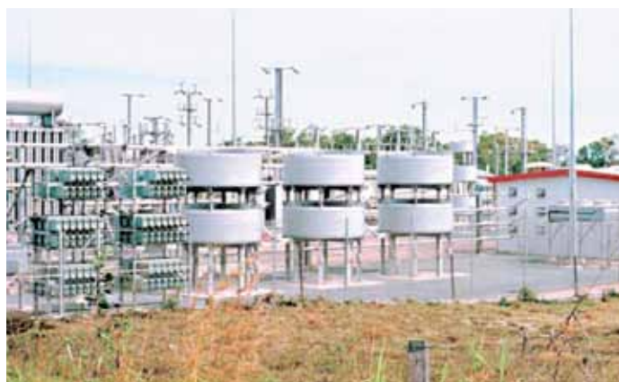
Oonoie SVC: 132 kV, -41/+52 Mvar
