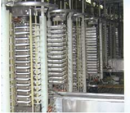
Fig. 3. SVC Light IGBT valve assembly.
