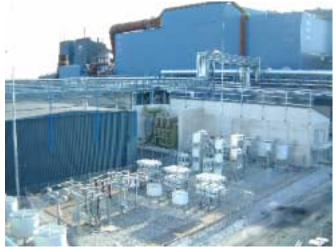
Fig. 2 The AvestaPolarit SVC Light installation.
