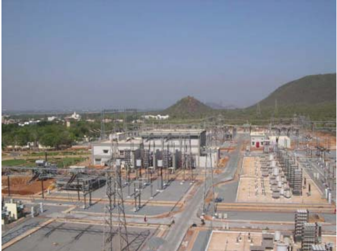
Figure 5.0 View of Second 1 x 500 MW HVDC Block from South Side
