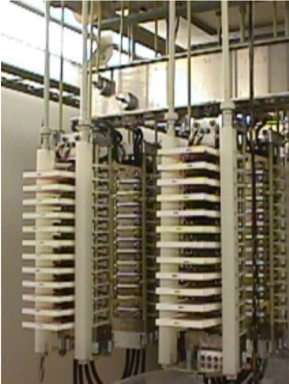
Fig. 8. Photograph of IGBT stacks.
