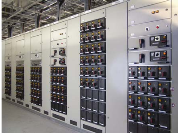
New 380V power controller cabinets
