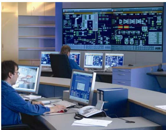
View from the chief unit operator's desk onto the Unit 4 control room
