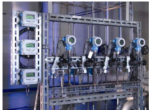
New transducers on the existing measuring rack
