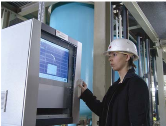
Local operator console in the condensate-polishing plant
