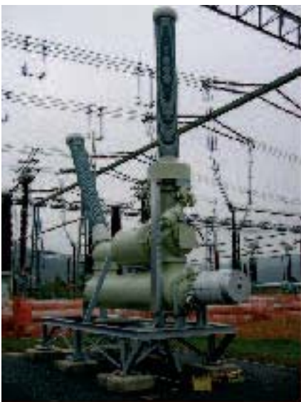
The new 380 kV hybrid switchgear
