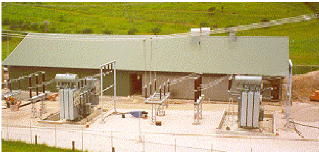
Fig. 8 shows one of the two converter stations in Directlink
