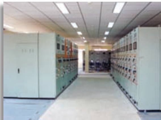
220/132/33 kV Control and Relay Panel
