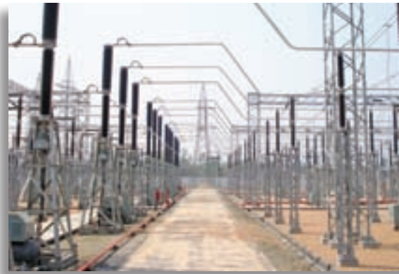
220kV Bus Bar System and circuit Breakers
