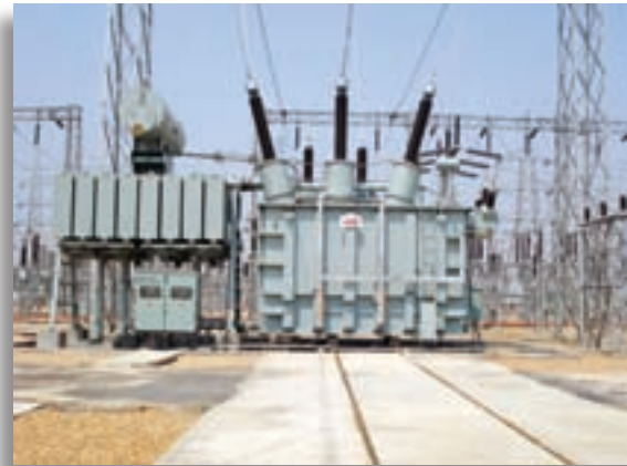
220/132/33 kV 160 MVA Power Transformer
