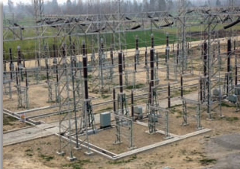
220 kV Circuit Breakers and Current Transformers
