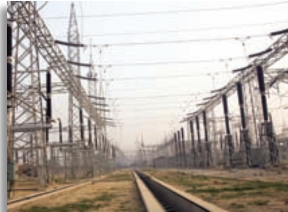
220 kV Circuit Breakers and Disconnectors
