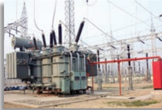
220/132kV 100 MVA Power Transformer with Fire Fighting System
