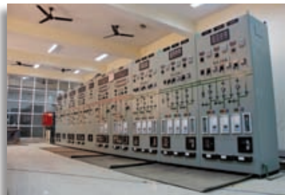
220/132/33 kV Control and Relay panels
