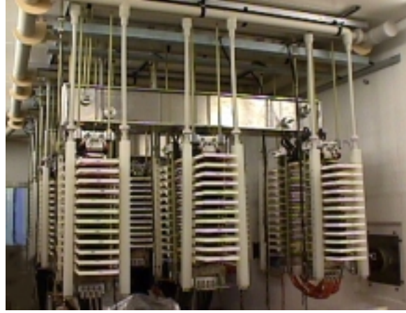
Fig. 6: SVC Light valve assembly.
