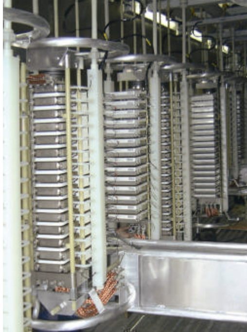
Fig. 5. SVC Light valve assembly.
