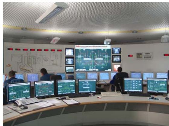
Control room of the Ruhleben waste-incineration plant
